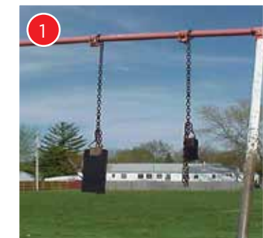
Swing chain should be unwrapped/inspected and broken swing seat should be replaced.
