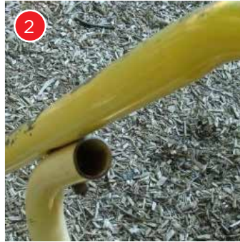
2 The cap is missing and should be replaced.
